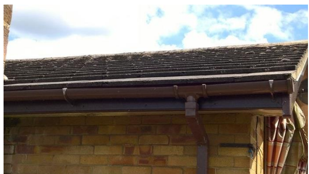
Plate 4.3: Raised Roof Tiles on Northern Elevation of No. 78 Tatenhill Lane.
