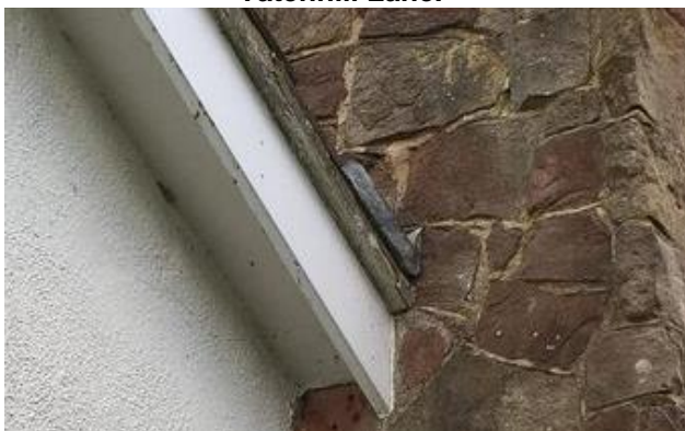
Plate 4.9: Gap Between Chimney Stack and Lead Flashing.
