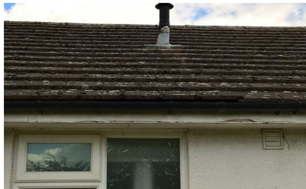
Plate 4.8: Lifted Tiles Around Guttering on the South-western Elevation.
